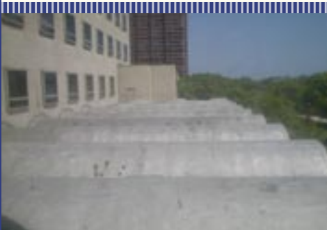
"Before" picture of scalloped roof.
