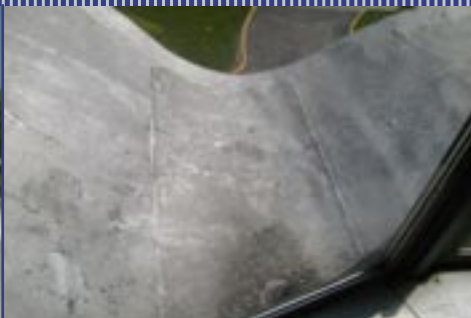
"Before" picture of aged valley in roof.
