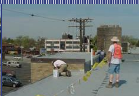
Steel foam stop manufactured by our sheet metal dept. was installed along the roof perimeter.
