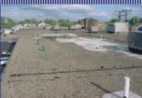
Ponding water is clearly visible in this "before" picture.
